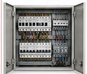
20 POWER DISTRIBUTION PANEL
