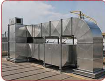
2. INLET & EXHAUST DUCTS
